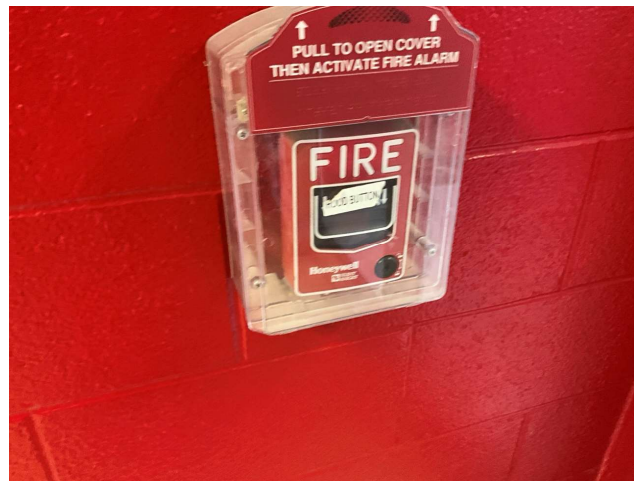
28 - FIRE ALARM SYSTEM
