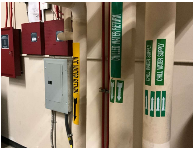
21 - HVAC HYDRONIC SYSTEM
