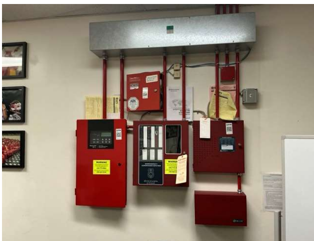
29 - FIRE ALARM PANEL
