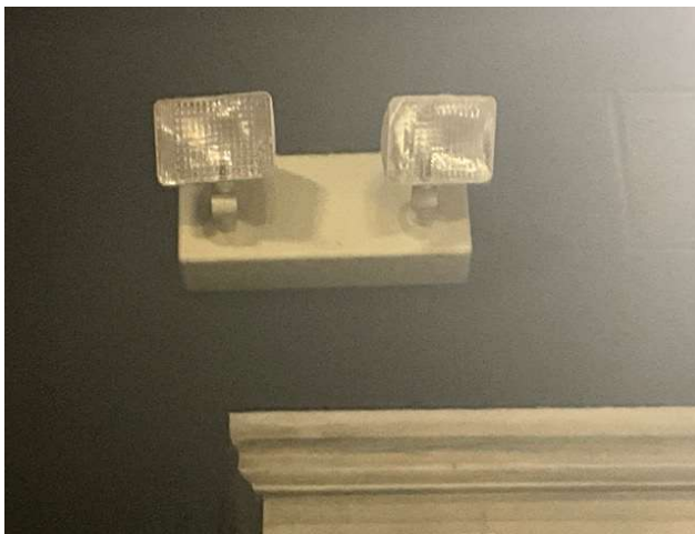
27 - EMERGENCY & EXIT LIGHTING SYSTEM
