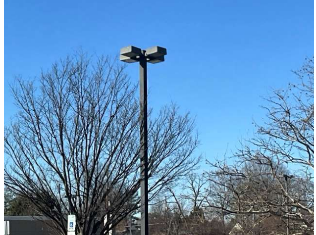
38 - PARKING AREA LIGHTING
