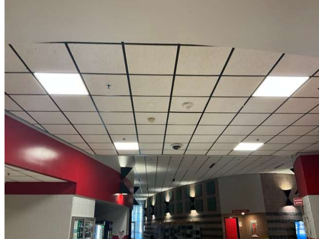
26 - INTERIOR LIGHTING SYSTEM
